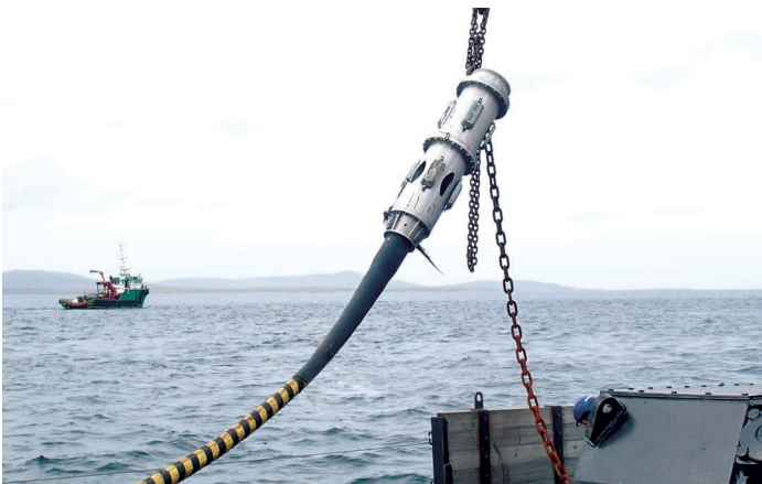
▲ MacArtney ILT connects a tidal turbine to the grid (image courtesy of Andritz Hydro Hammerfest).
